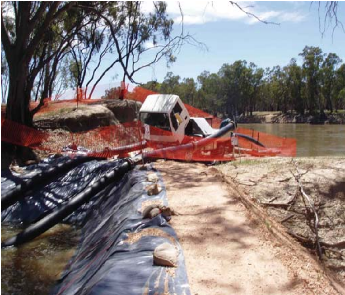
Figure 1: Mobile pumping infrastructure used to deliver water to the Hattah Lakes Icon Site (Photo: Murray-Darling Basin Commission).
